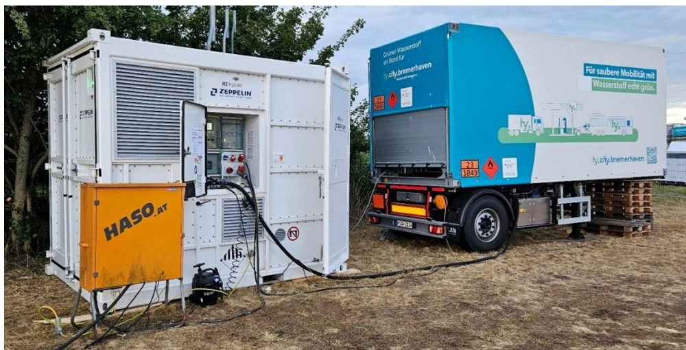
Zeppelin Power Systems' PEM demonstrator in practical use
