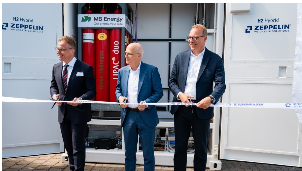
Inauguration of the fuel cell power generator from Zeppelin Power Systems: The hybrid PEM demonstrator combines a fuel cell with battery storage and enables an emission-free, decentralized power supply
